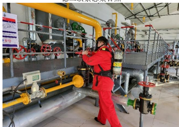
应急泄漏检测
